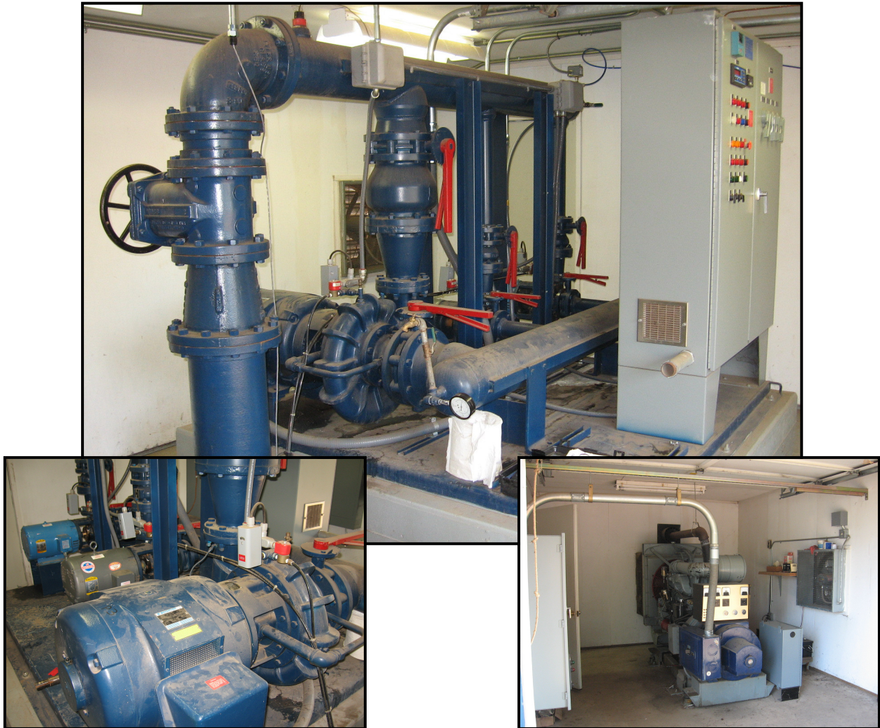
Figure 2 – 9 Booster Pump Station
