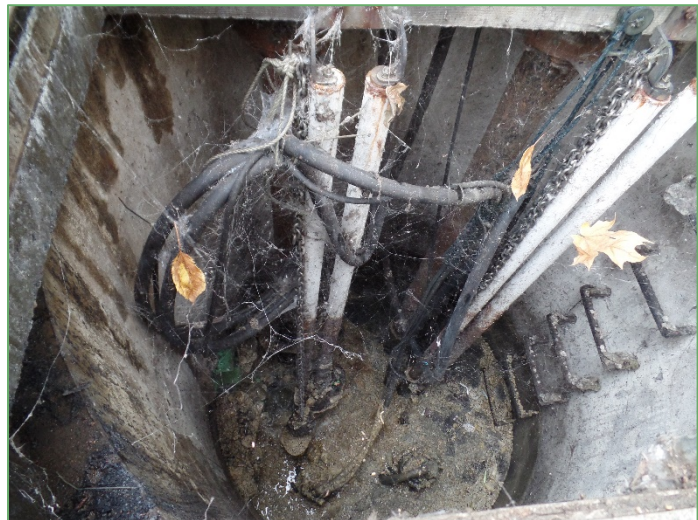
Lift Station 2 Wet Well
