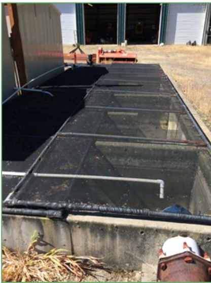
Chlorine Dosing System
