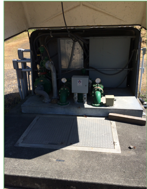
River Pump Station / Irrigation Pump Station
