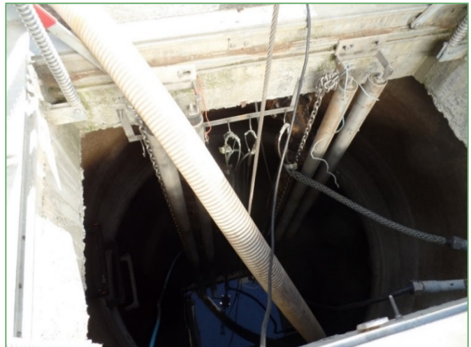
Return Pump Station
