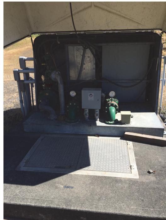
River Pump Station / Irrigation Pump Station
