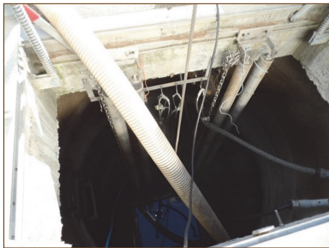
Return Pump Station
