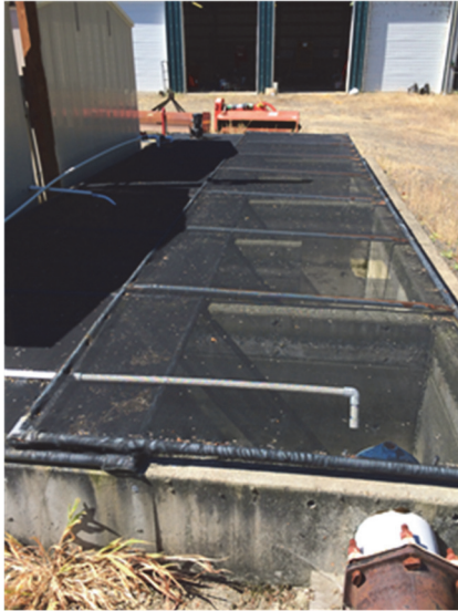
Chlorine Dosing System
