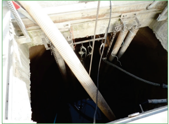
Return Pump Station
